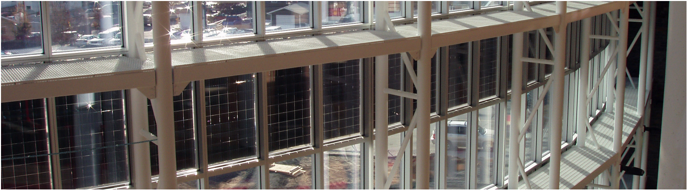
Interior view of south facing VISIONWALL® BIPV curtain wall system
